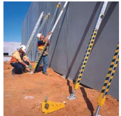
3. Attach the foot of the brace to the brace anchor and fix the head of the brace to the precast concrete panel.
