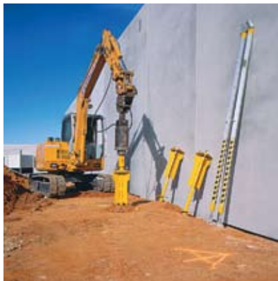
2. Install each brace anchor where marked anytime before erection of the precast concrete panels.
